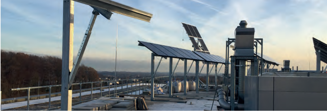
New photovoltaic installation on the roof of the Bielefeld Fachhochschule
