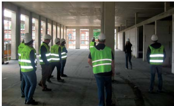
End of structural work: first construction site visit for students of architecture, civil engineering and construction project management (Source: U. Schramm, May 16, 2014)
