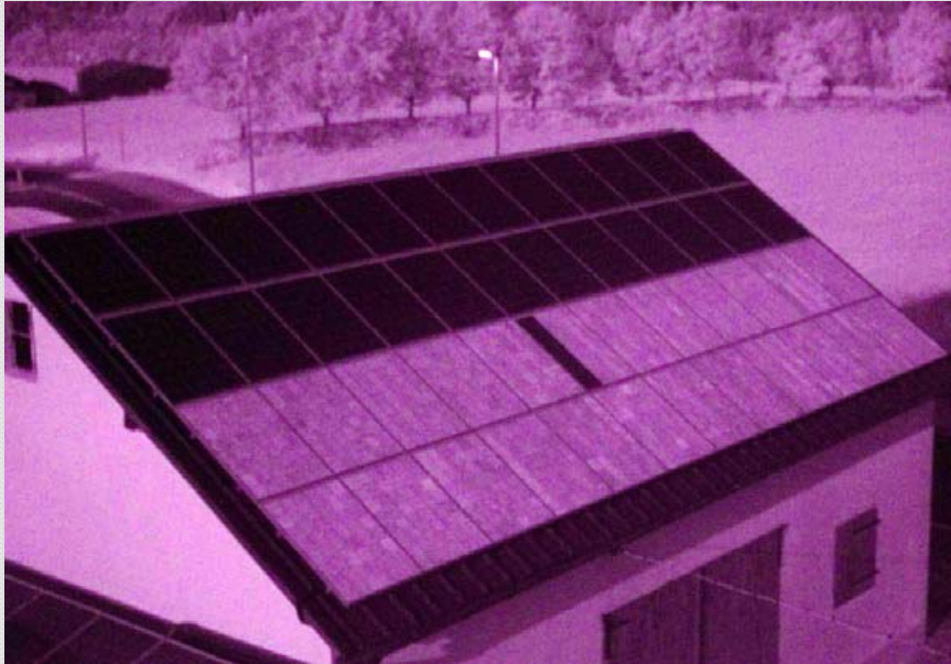
Detection of defect by-passdiode
